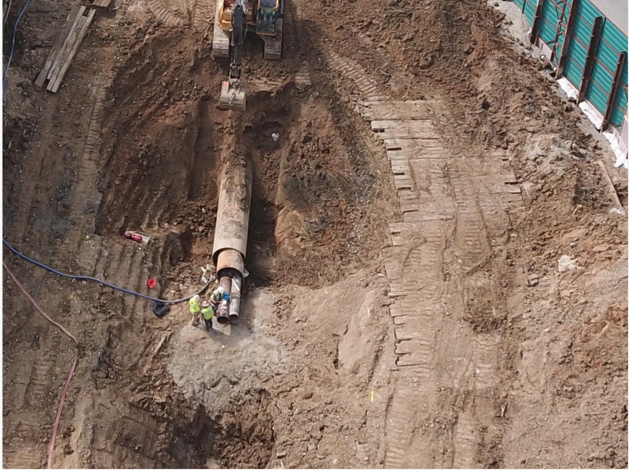
Mariner East pipelines lying next to each other within a casing in Edgmont Township after HDD pipe “pull back”.
