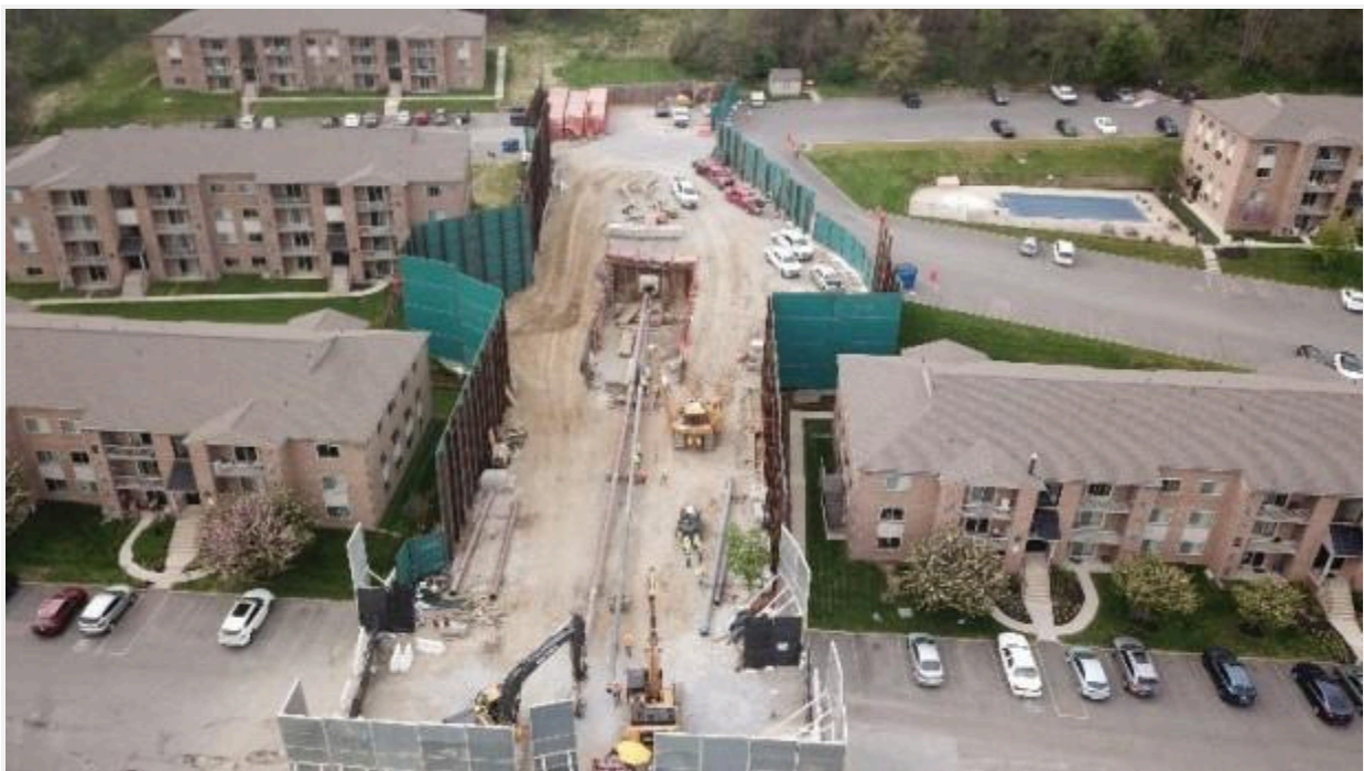
Mariner East pipelines lying dangerously close to each other during pipe "pull back" at Glen Riddle Apartments in Middletown Township.
